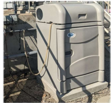
Figure 10. Final Effluent Sampling Location
