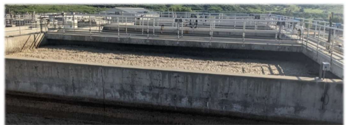
Figure 5. SBR Basin Sampling Location
